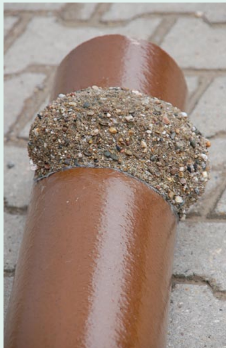
Resin leakage at damaged area
