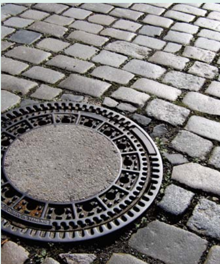
Manhole cover: the visible interface with the drain and sewer system photo: unikation, photocase.com
