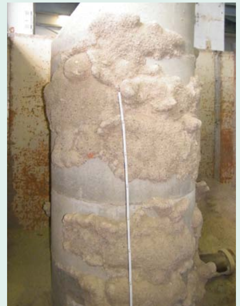
Figure 2: Repair methods in IKT projects: manhole sealing – injected polyurethane on the manhole exterior
