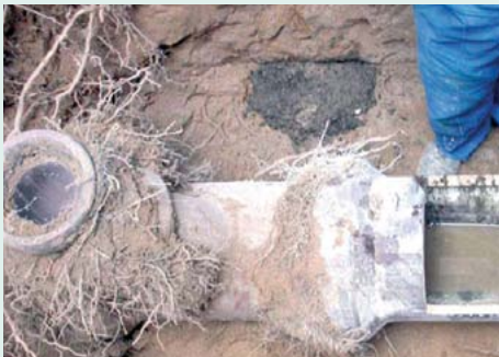
Figure 3: Excavated pipe penetrated by roots
