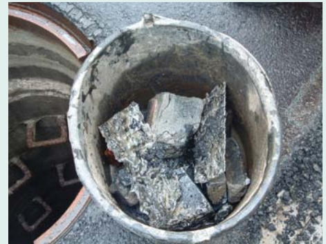
Building rubble causing obstruction to flow: after-completion inspections may be appropriate in the zone around completed civil-engineering work.
