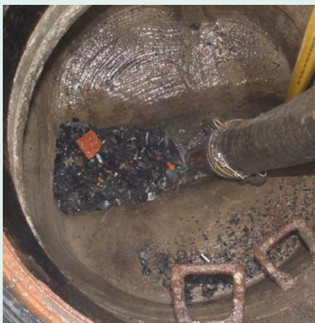
Recurring problems: Knowing where depositions regularly occur permits systematic cleaning.
