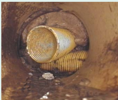
Illegal drainage system connection to a public sewer source: Municipality Möhnesee
