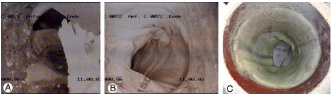
Figure 6. Examples of visually unsatisfactory repair results on extreme damages A Robotic system - view from the main pipe. B Top hat liner - view from the main pipe. C Top hat liner - view into the connecting pipe (after disassembly).
