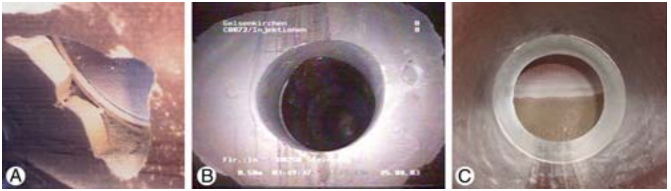
Figure 2. Standard damage for robotic systems and example of a visually satisfactory repair result. A Initial situation. B View from the main pipe. C View into the connecting pipe.
