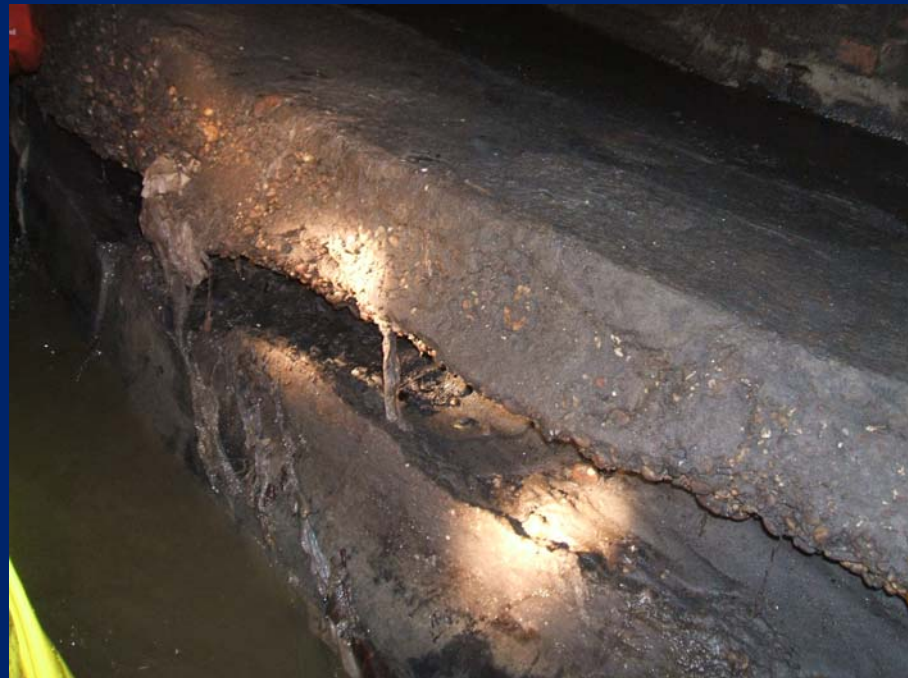
Sags with inclination (bedding material flushed out)
